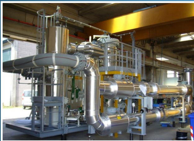
VOLUMETRIC METERING DN 10" # 300 RF
