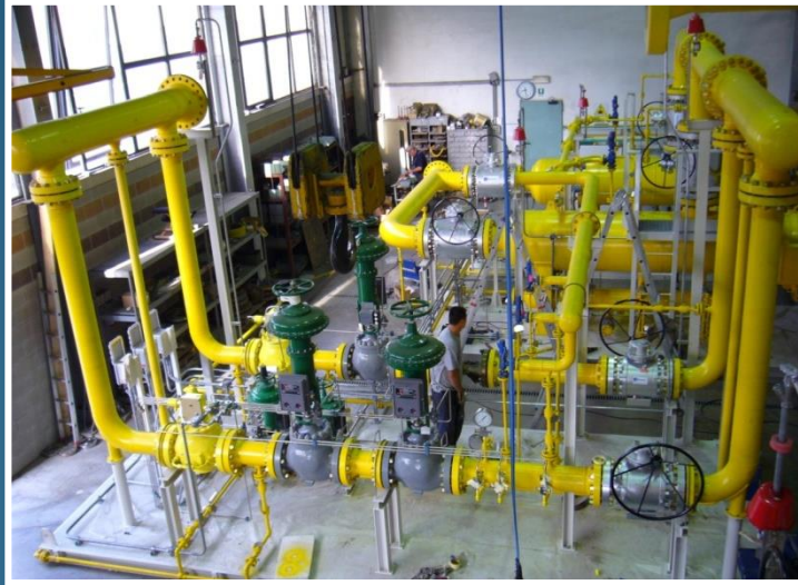
PRESSURE REDUCING 48÷36 bar. FLOW 70.000 NM 3 /h, 14" PIPING
