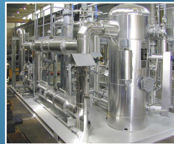
FUEL GAS PACKAGE FOR GAS INJECTION STATION # 300
