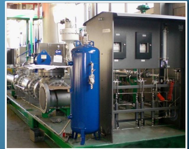
FISCAL METERING DN 14" # 600 RJ
