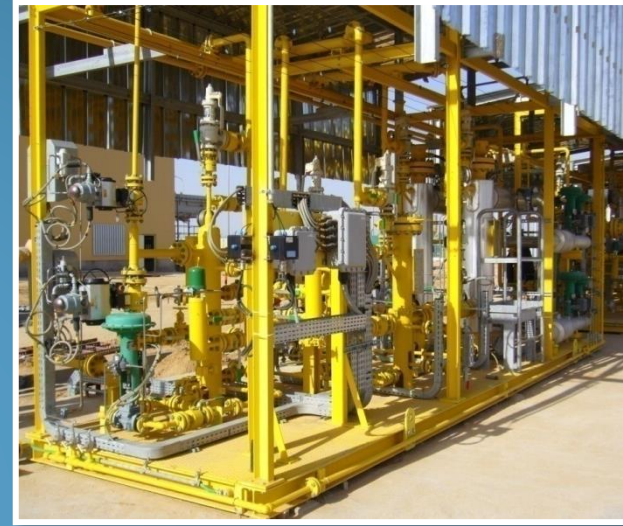
PRESSURE REDUCING 62÷20bar. FLOW 2.250 NM 3 /h, 3" PIPING
